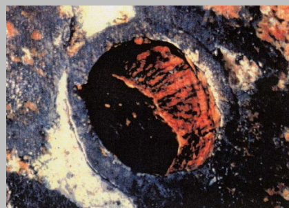
Microbial corrosion in a tank
